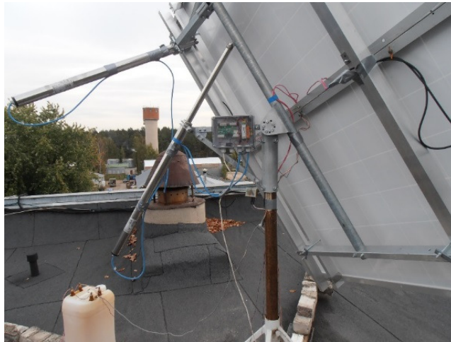
Fig. 1. Solar tracking device ST44M2V4P with two push bars and two solar photovoltaic panels Solet P6.60-WF-250
